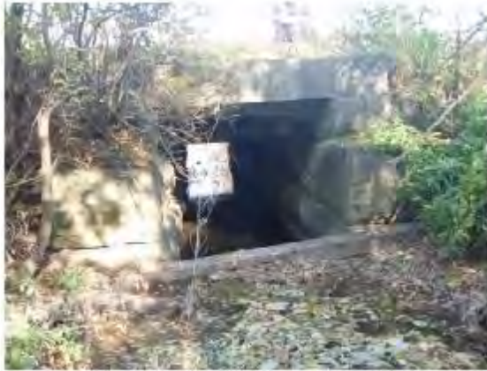
GRADE CONTROL AT CN CULVERT CREATING BACKWATER CONDITIONS
